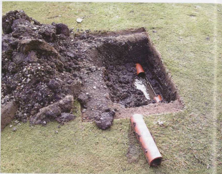
▲ Old fairway drains may need replacing with more appropriate and effective modern drainage systems.
