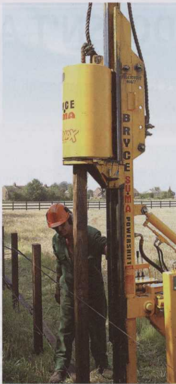
A ram is the fastest way to accurately sink posts at a consistent depth with level face for the rails.
