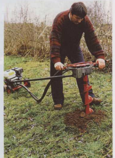
This one man earth auger takes the hard work of making post holes.
