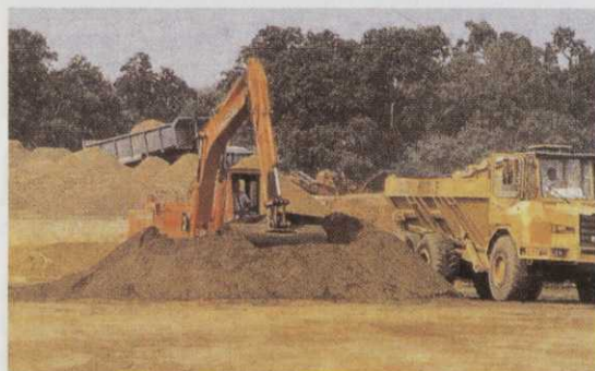
Mixing root zone of fen soil and sand is best done centrally, off site.
