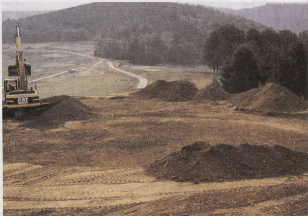
Mixing on site should never occur.
