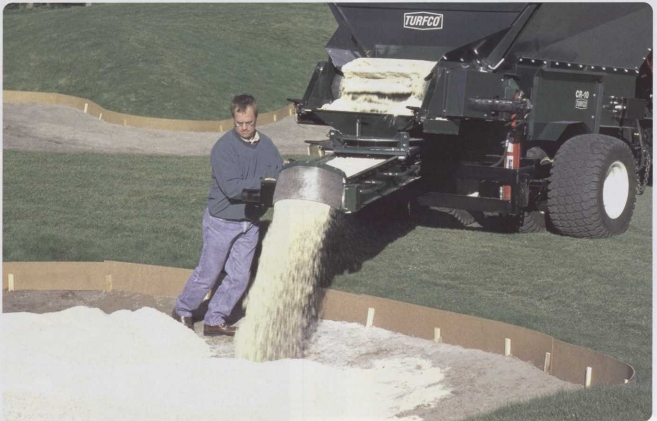
Below: The cross conveyor with swivel action deposits materials exactly where they are needed
