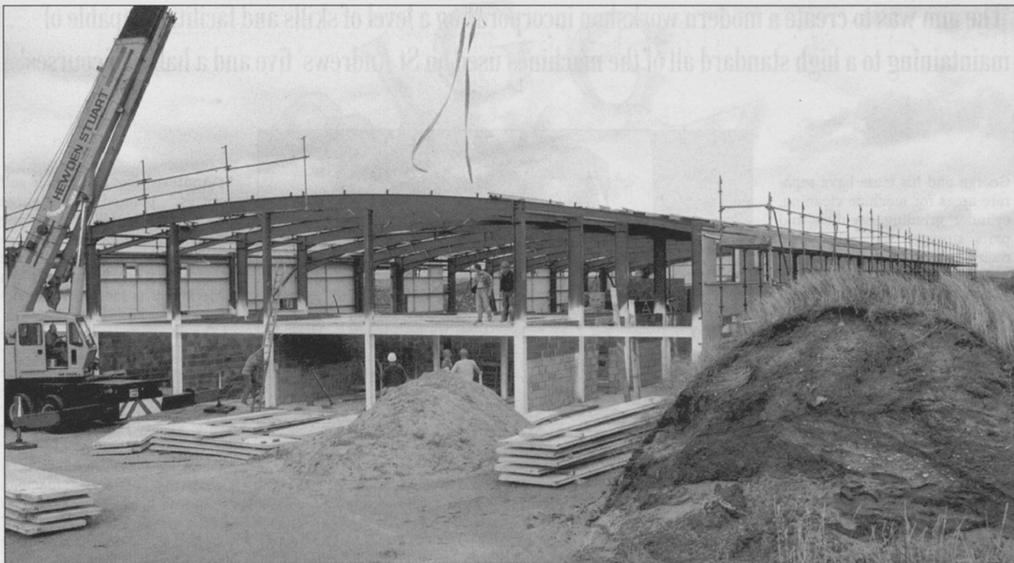
The Jubilee Greenkeeping Centre under construction last year: Staff facilities and administration wing are laid out on two floors at the southern end of the building
