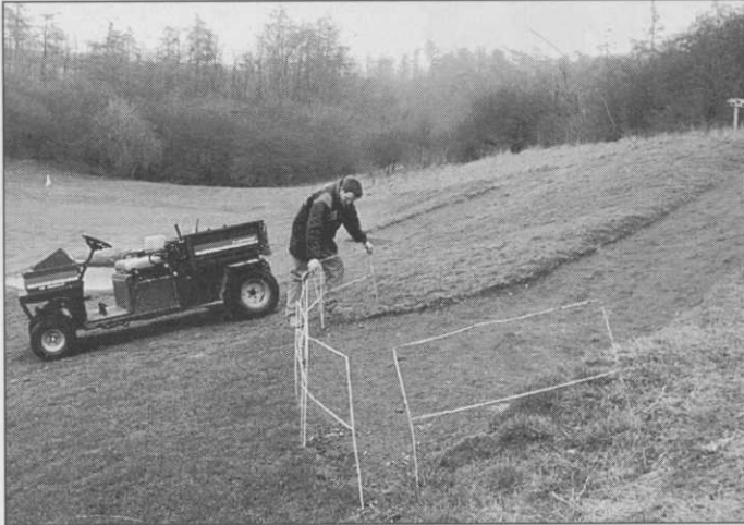
Ground under repair. Returfed areas must be protected from golfers, trolleys and course machinery. Note alternative routes from the green to the next tee
