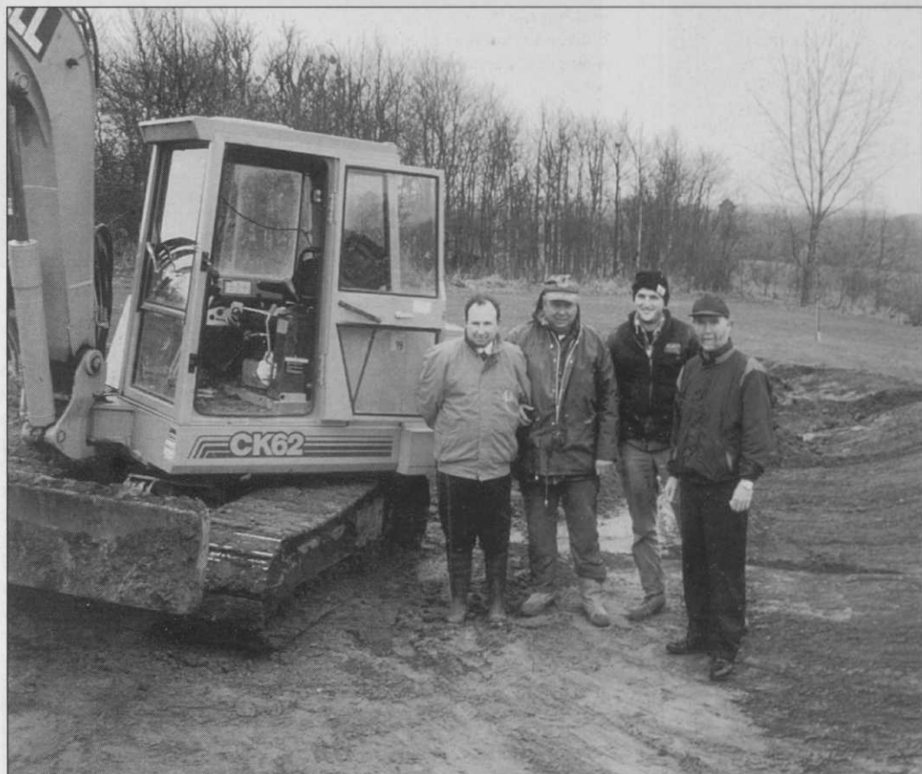
Ian Scott Taylor, left, and Bill Sparrow, right, with two members of Cousell Associates Ltd construction team
