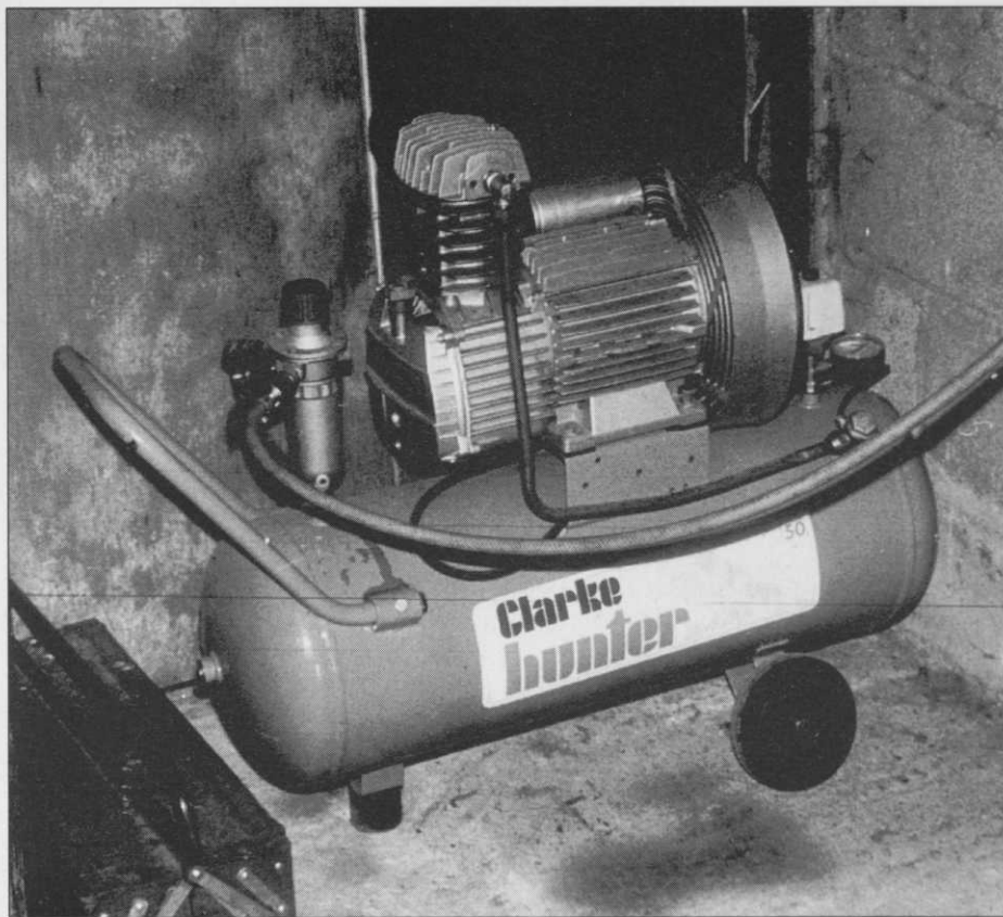
A Clarke Hunter compressor and air receiver at Earlstoke Sands
