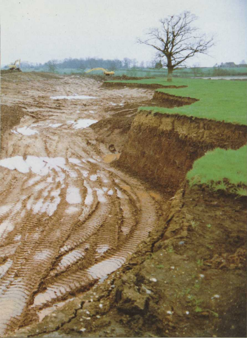
Pond under construction: clay seals are not necessarily easy to form. Vertical faces require special treatment
