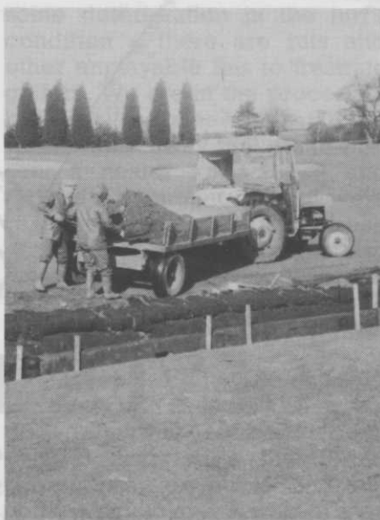
The bank of a ditch is improved for a smart appearance and to ease maintenance.
