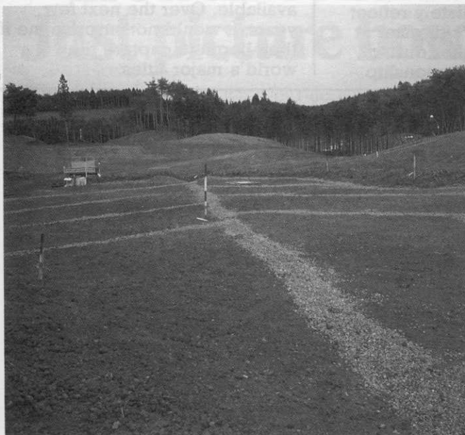
Greens drainage follows the USGA specification.
