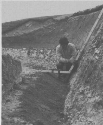
Bank shaped and base ready for first row of turf. A wooden frame was constructed to maintain the correct wall face angle.
