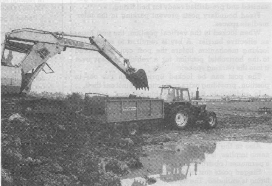
Construction of a new 18th green and practice putting green at Weymouth, showing the problems of working a heavy clay site in wet weather.
