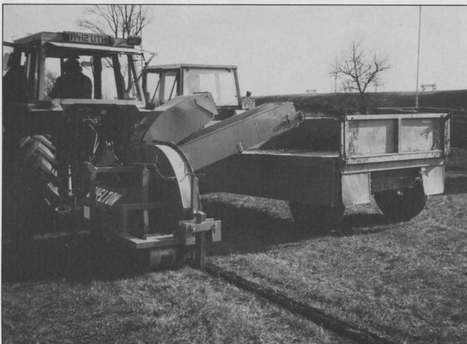
A tractor operated super-trencher cuts a 2" wide trench. The excavated soil can be used on other parts of the course
