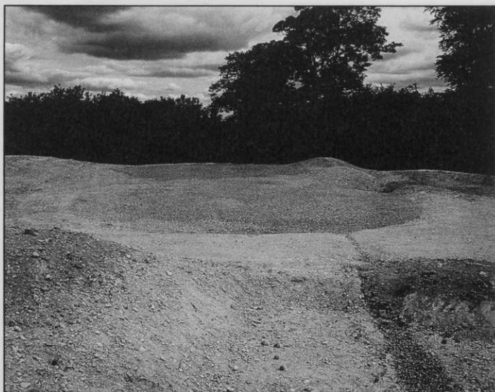
Early stage of construction to the 2nd green, showing the stone base.
