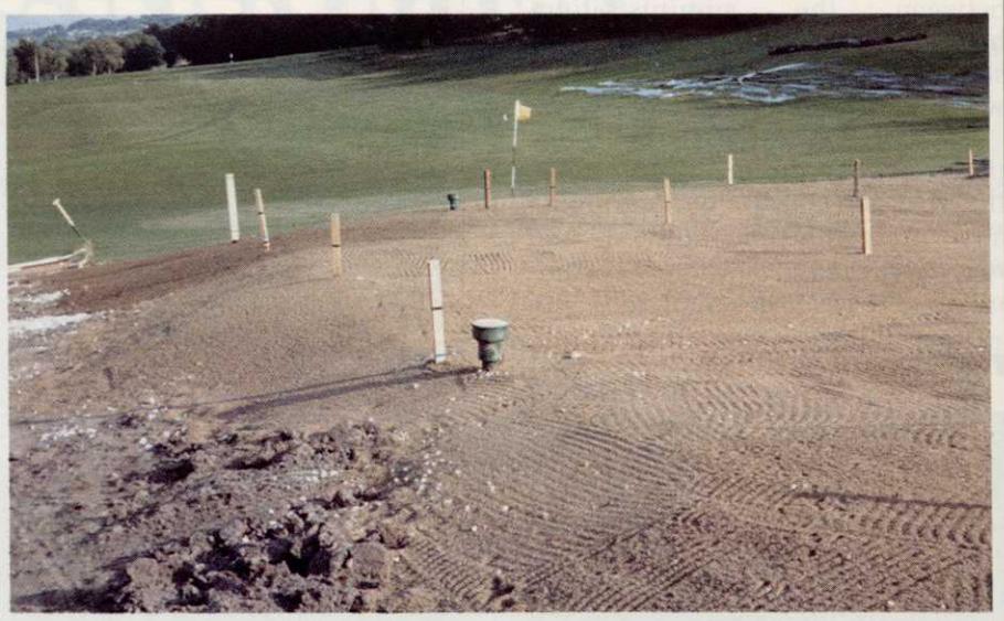
Drains and stone carpet completed. Sharp sand laid to a depth of two inches, ready for the nine inches of top mix. Note the marker posts at 12 foot centres with coloured bands showing the level to be achieved. The flag post for the temporary green can be seen in front of the workings to allow play to continue throughout the month.
