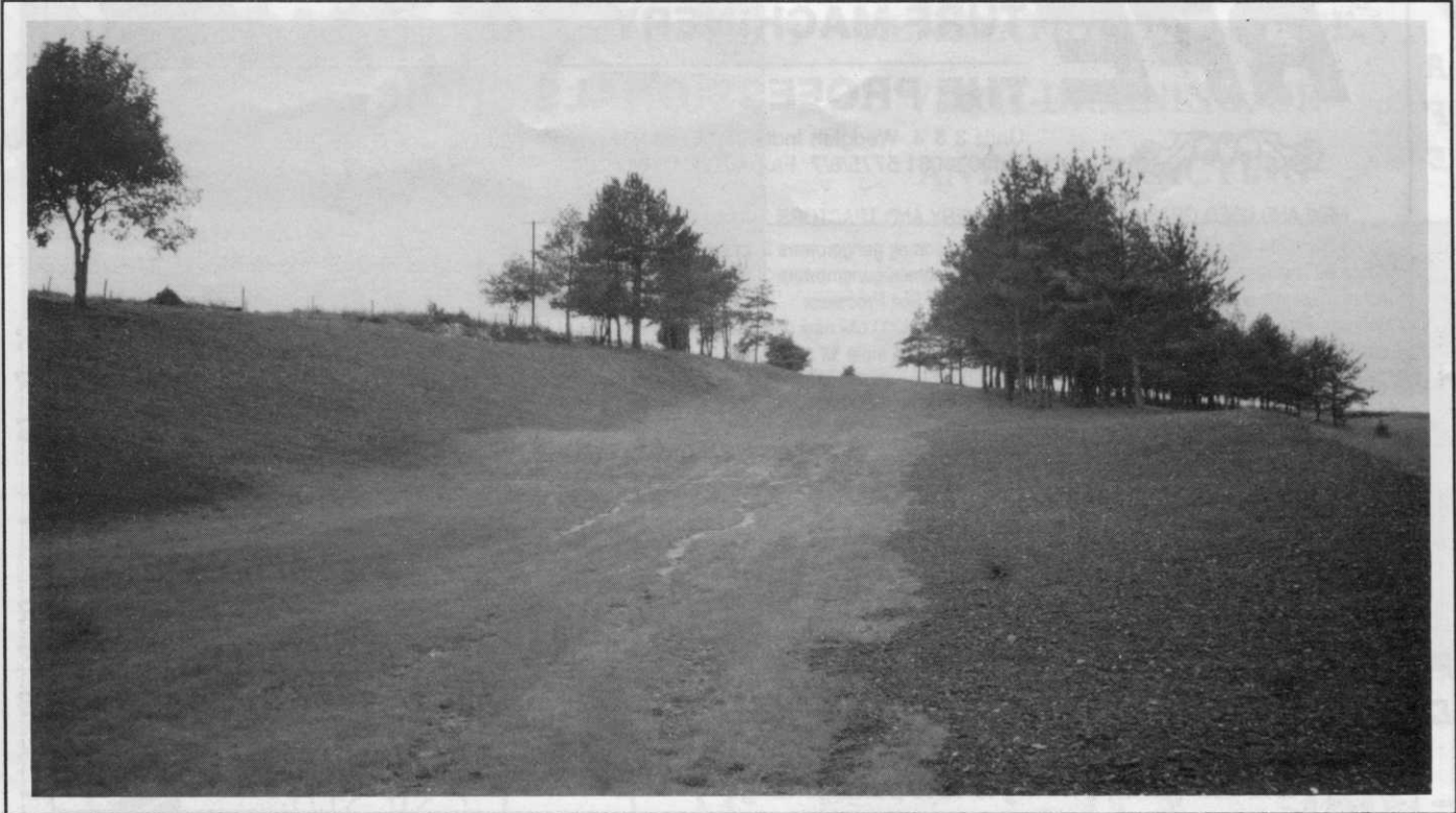
View of fairway from a tee shot landing spot. The position marked by small bush on horizon between gap in the trees. Exposed soil left and right is where features were modified this autumn to enlarge playing surface width.
