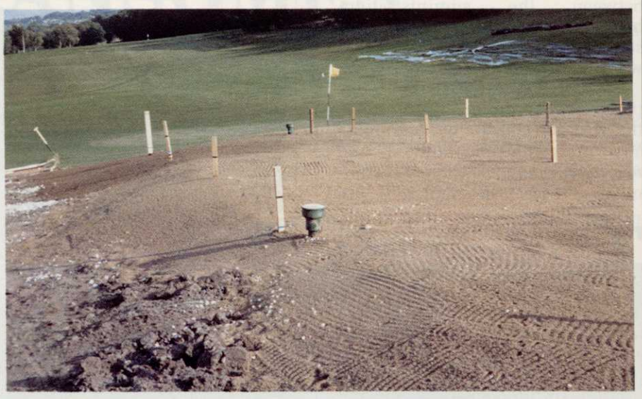
Drains and stone carpet completed. Sharp sand laid to a depth of two inches, ready for the nine inches of top mix. Note the marker posts at 12 foot centres with coloured bands showing the level to be achieved. The flag post for the temporary green can be seen in front of the workings to allow play to continue throughout the month.
