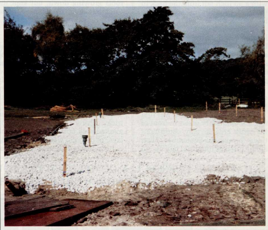
Hard limestone used in the re-construction of the fifth green at Shipley.
