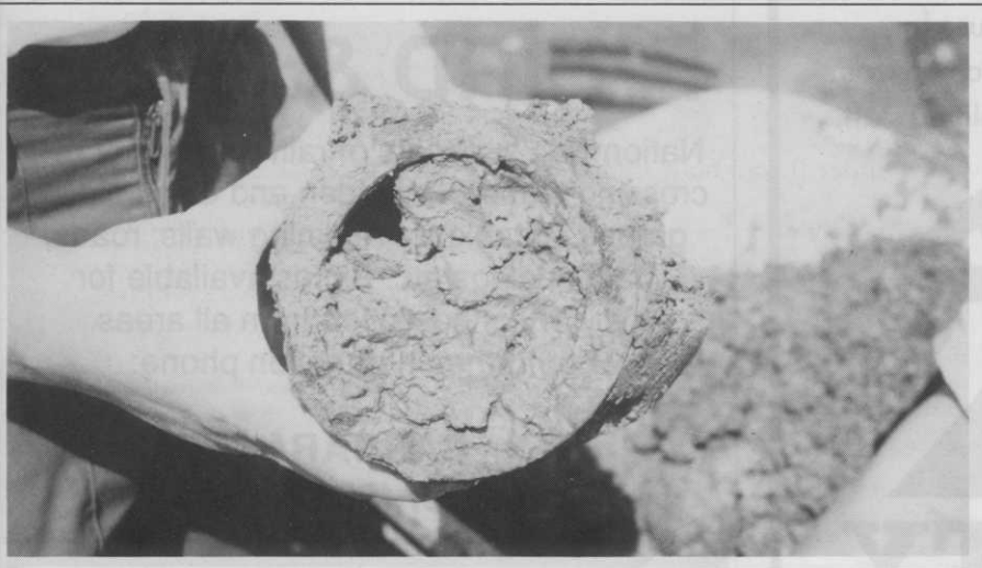
Old drain of green 4
