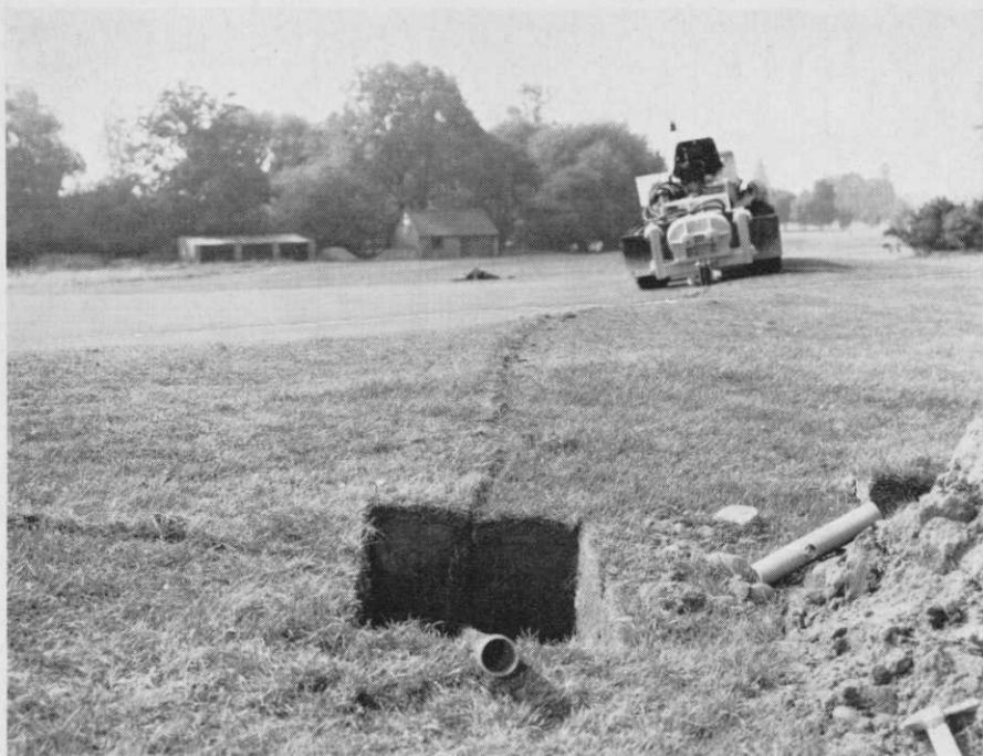
Mole ploughing supply pipe around a green. Note the negligible disturbance of the turf. Photograph: Wright Rain Limited
