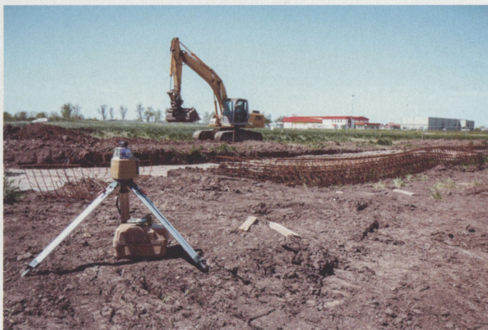
Most contractors suggest purchasing skid-steers or mini excavators if you plan to use them a handful of times per year.
