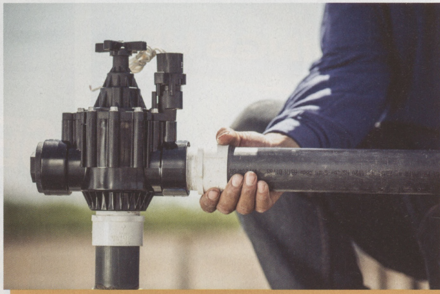
Routine maintenance and winterization can keep valves lasting a long time.
