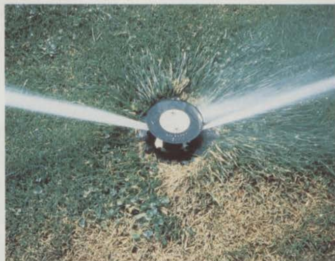
All sprinklers need to be adjusted for distance and arc each year.
