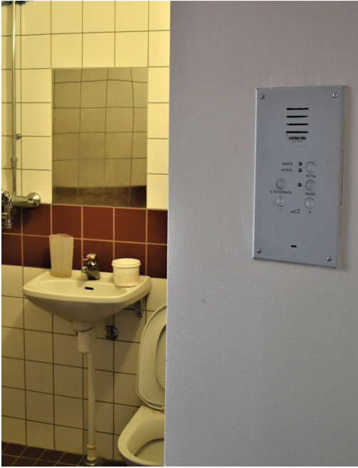
Figure 10.24 Cell intercom system, Helsinki Prison, Finland
