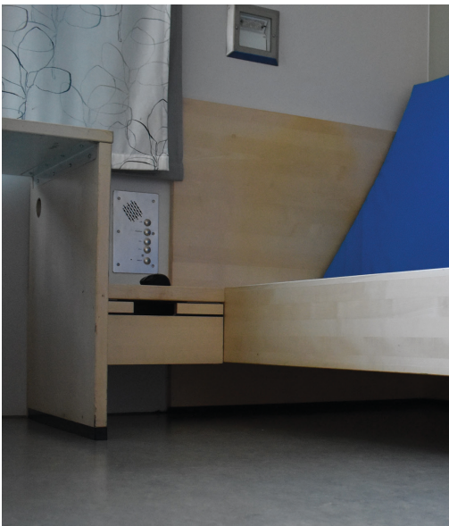
Figure 10.25 Cell intercom system, Halden Prison, Norway
