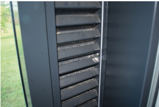
Figure 10.23 Close-up of the air intake on one side of the cell window, Halden Prison, Norway
