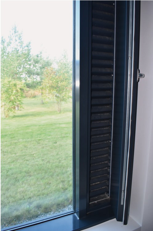
Figure 10.22 Air intake on one side of the cell window, Halden Prison, Norway
