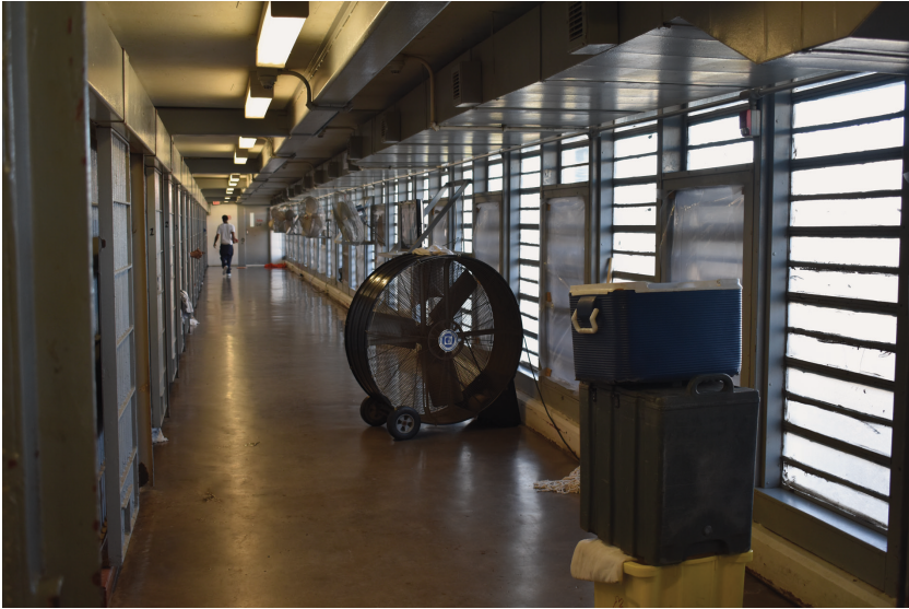
Figure 9.14 Louisiana State prison “Angola” Camp A. Corridor and a row of cells (left) in front of translucent polycarbonate windows for contact with daylight (right)
