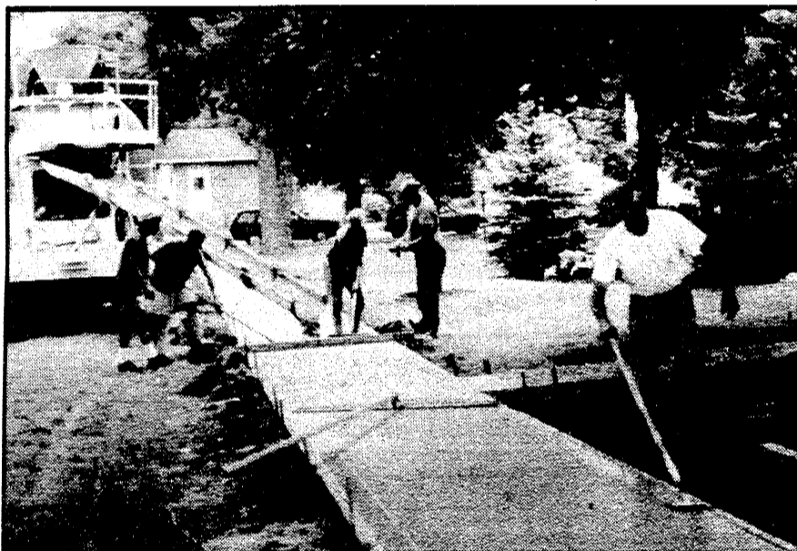
The job of smoothing the concrete begins. A sidewalk also extends to the home of Ron & Susan Fielder, who requested the sidewalk be installed. Sue Fielder is a member of the Parks Commission and maintains an avid interest in upgrading our Village's recreational property.
