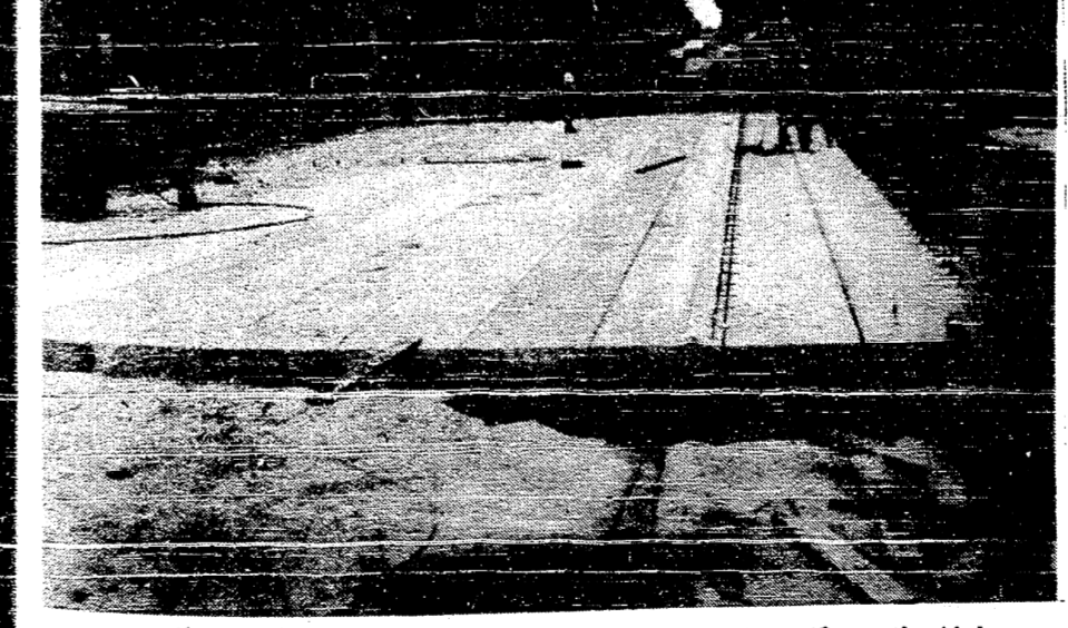
The final beam was lowered into place, Tuesday, June 13, on the Main Street bridge. With three weeks to go, completion is right on schedule.
