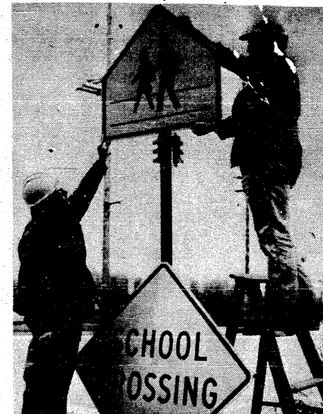
THE OLD AND THE NEW--All over Michigan, new symbol signs are gradually replacing traditional word signs under a nationwide highway safety signing program. Here, sign technicians H. R. Warren (left) and Tom Jancke of the Department of State Highways take down a school crossing sign and replace it with the new yellow and black symbol sign conveying the same cautionary message. (Department of State Highways photo)
