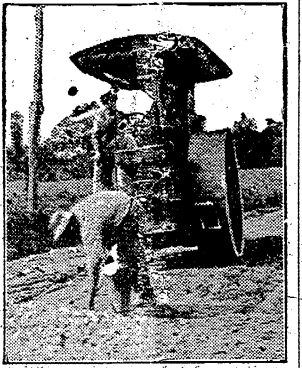
Building a Hard Rock Road. amounting to $250,000 had been allotted to Dallas county for its high-
