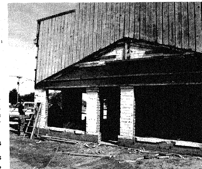
GOING DOWN: The former Performance Ford building on the southeast corner of M-25 and Bay Street south of Sebawaing was razed last week. Kemp Land Improvement Contractors did the work, as shown here.
