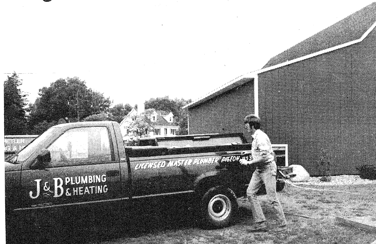
WORK CREWS from J & B Plumbing and Heating and Shetler Plumbing and Heating were busy at the Band Shell on Saturday.
