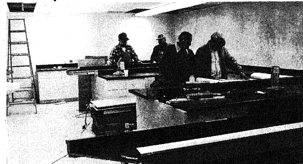
Project Manager Lex Tetreau, center, looks over blueprints in Scheurer Hospital's new laboratory, under construction.
