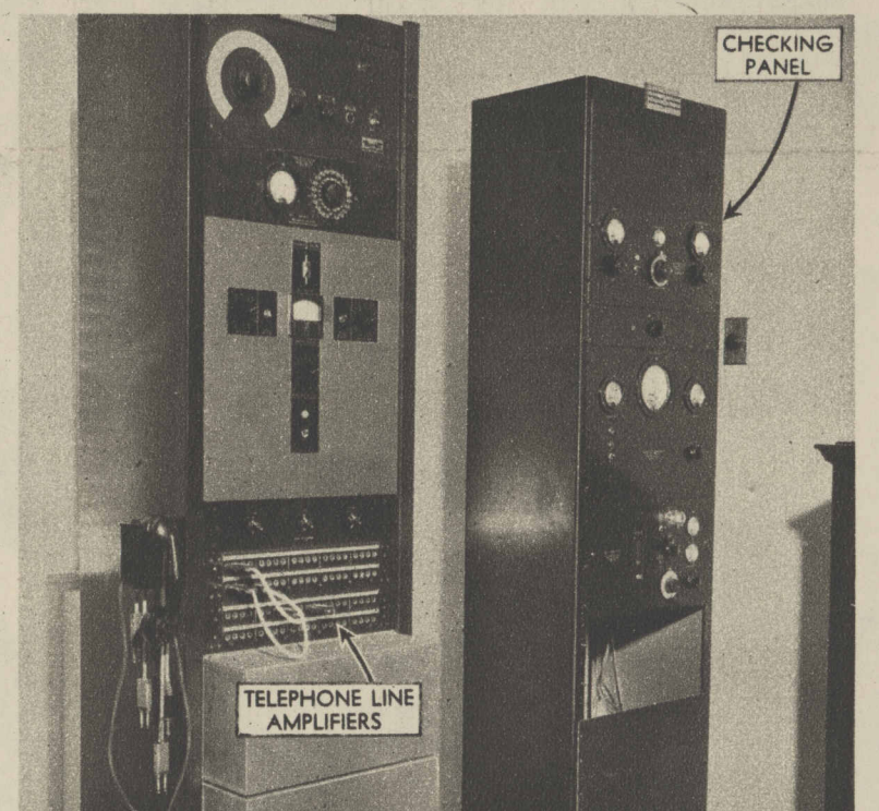
Telephone amplifiers through which pass electrical impulses carrying program from W-G-N studios. Checking panel is used to keep tab on equipment.
