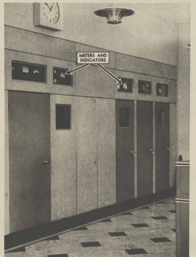
Transmitter front panel. Behind doors are giant tubes used to amplify power. (Tribune photos.)
