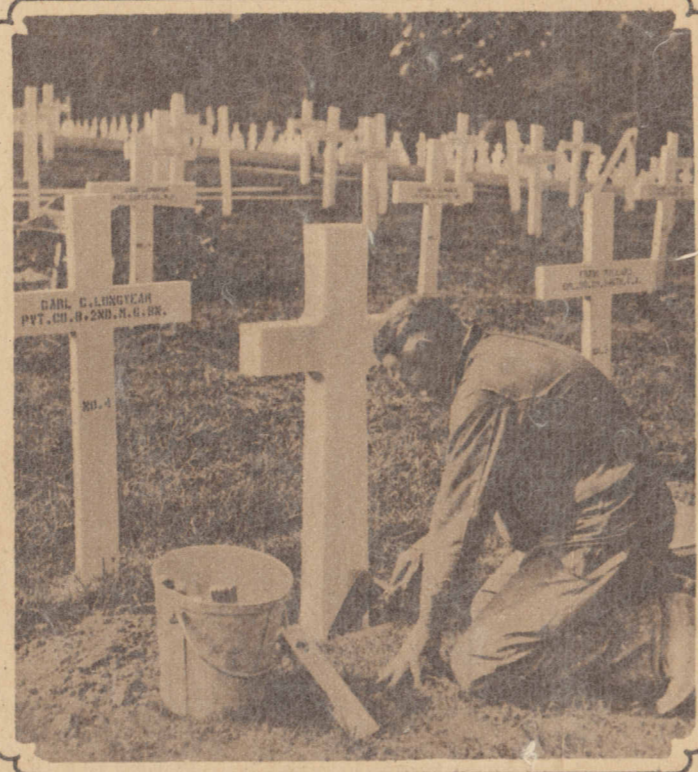
MARBLE CROSSES FOR YANKEE HEROES to replace the wooden ones over American graves in the cemetery at Surennes, France. Here a workman is installing one of the new designs. (Photograph from Wide World.)
