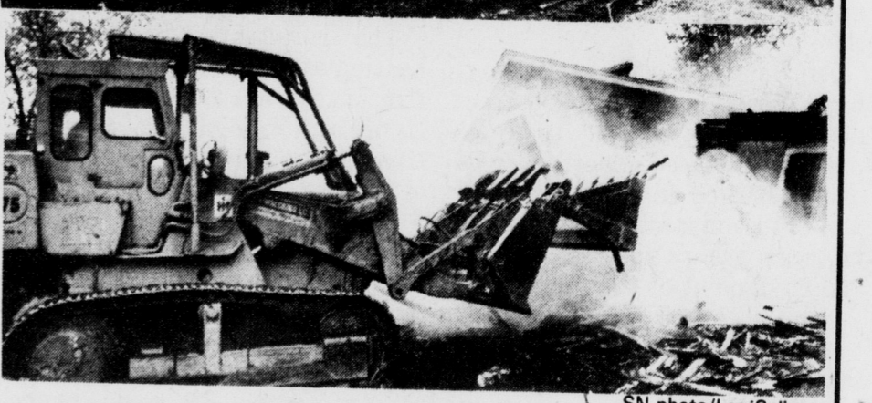
This house was demolished yesterday at the corner of M.A.C. Avenue and Ann Street as city officials make way for a 24-hour restaurant, offices and student apartments.
