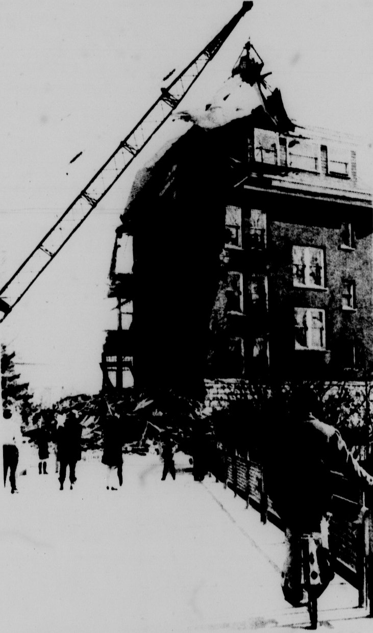
MAKE ROOM FOR THE LIBRARY--Even at 8:30 a.m. Saturday, students stopped to watch the demolition of Wells Hall, one of the oldest buildings on campus. A new addition to the Library will take its place. Photo by Chuck Michaels
