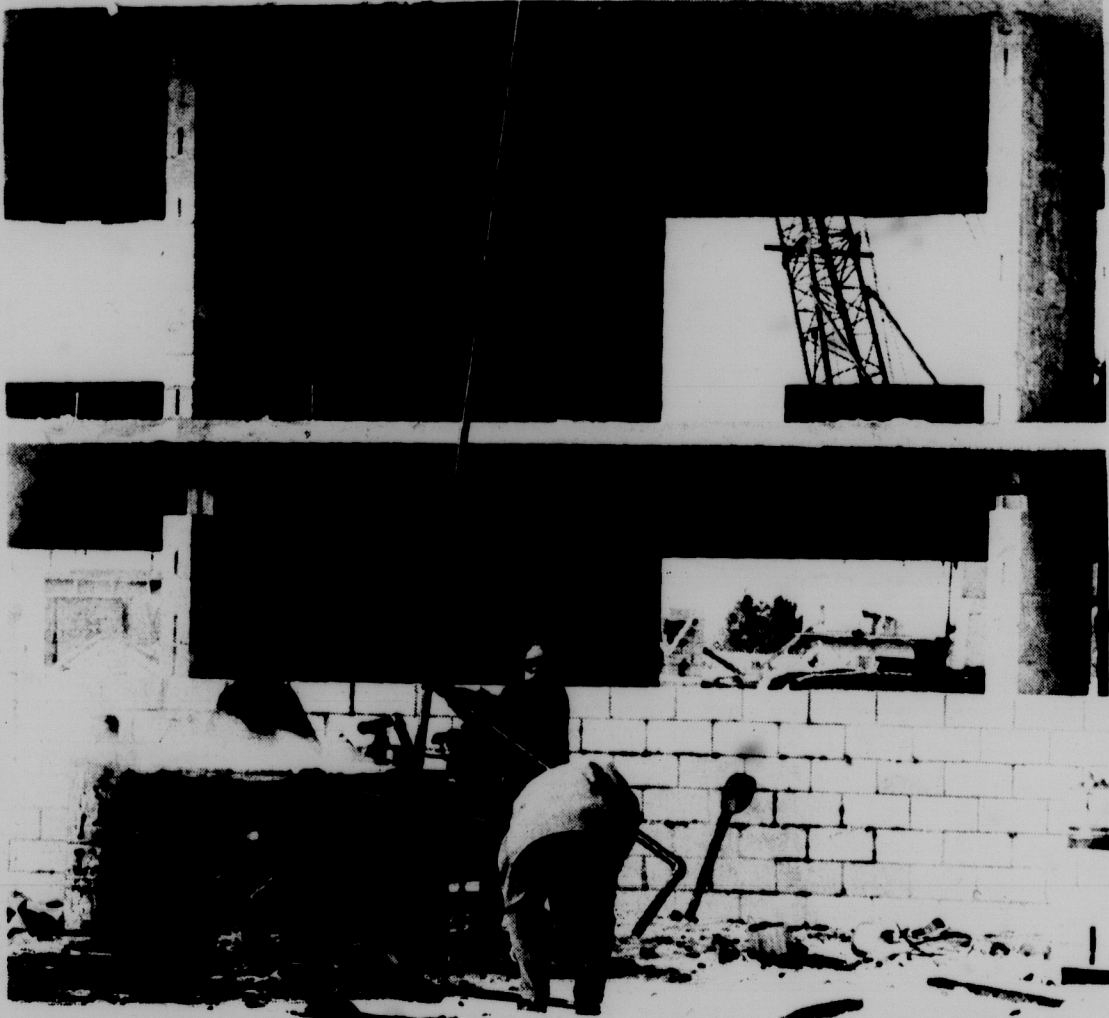
TOPPING 'EM OFF--They are getting their roofs this week, but the 228 apartments being built at Spartan Village won't be ready for married students until next summer. The $2 million expansion is on the southwest side of the village near the school. Photo by Tony Ferrante
