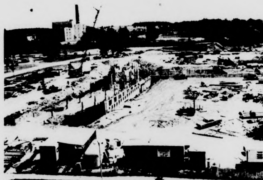
Shown above is a view of some of the foundation work being completed by the Granger Construction Company of Lansing. The tall smoke stack and building in the upper left corner of this picture is the newly operational Power Plant '65.
