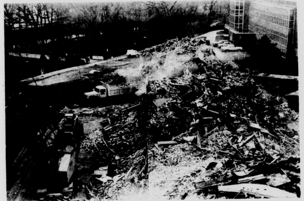
AFTER--What's left of Wells Hall waits to be towed away. This shot from the fourth floor of Olds Hall shows how much rubble an old office and classroom building and former dormitory can make. Photo by Chuck Michaels
