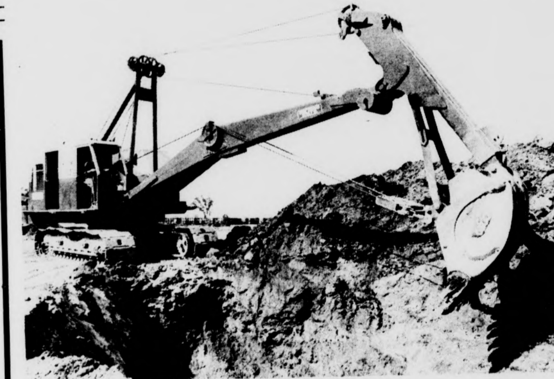
HEAVY CONSTRUCTION --Not an uncommon sight on campus is the appearance of heavy machinery to begin the construction on the many new buildings constructed each year. Here, a large earth mover breaks ground for start of a new building. Photo by Chuck Michaels
