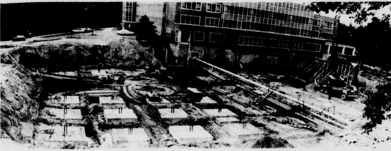
COMING UP--A long look at the graduate study library shows things beginning to rise. The expansion should add about 150,000 square feet of space to the library. Construction is scheduled to be completed Aug. 15, 1967. Photo by Tony Ferrante
