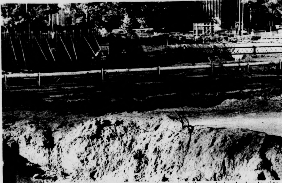
STARTING TO RISE--The big addition to the Main Library is beginning to rise from the big excavation where Wells Hall stood a few months ago. With the aid of a crane's long boom workers have started erecting sections of forms for the basement wall.
