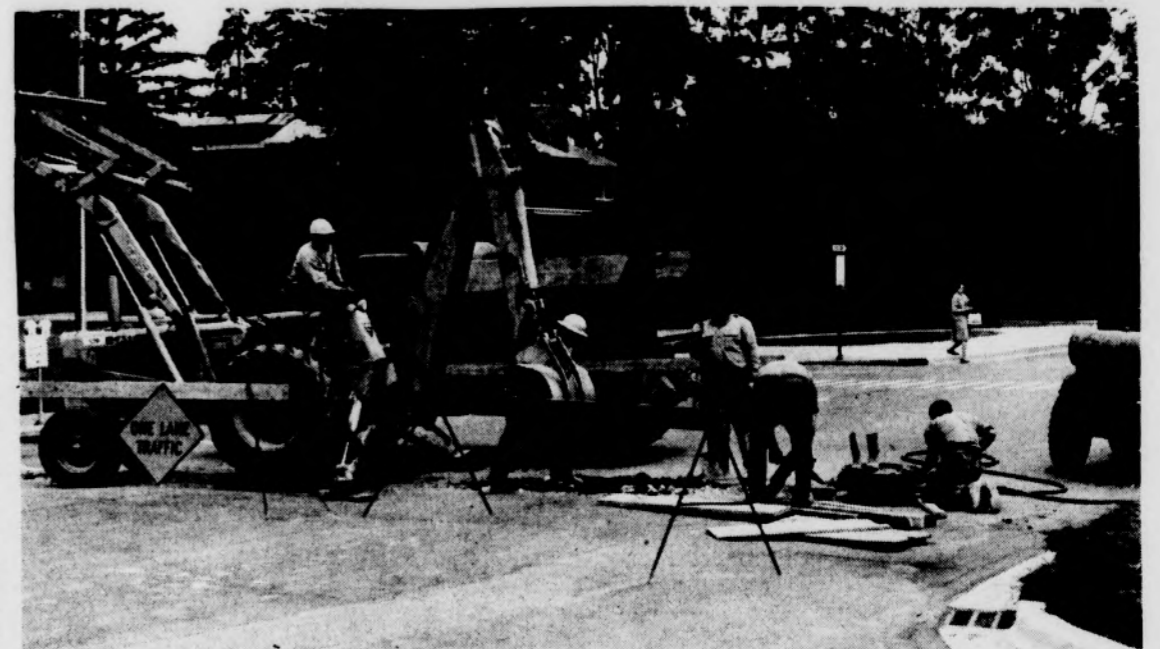
CONSTRUCTION OR OBSTRUCTION--Once again, workers are tearing up part of West Circle Drive. The work disrupted traffic most of the day. Photo by Russ Steffey
