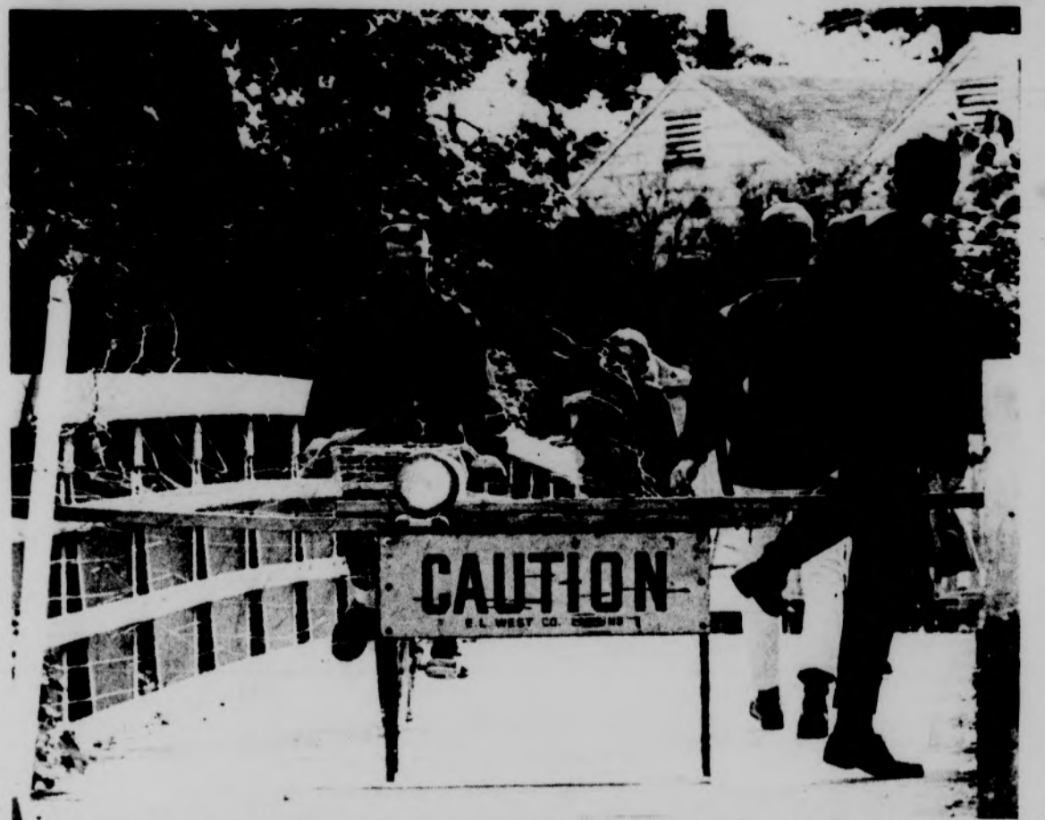
NOT A WAR ZONE--This photo is somewhat similar to those taken in riot-torn Dominican Republic. But it was actually taken near the new Language-Mathematics-Statistics Building site. Construction men will agree that baracades don't stop many students from a short cut. They do protect the company against damage suits, however. Photo by Larry Fritzman
