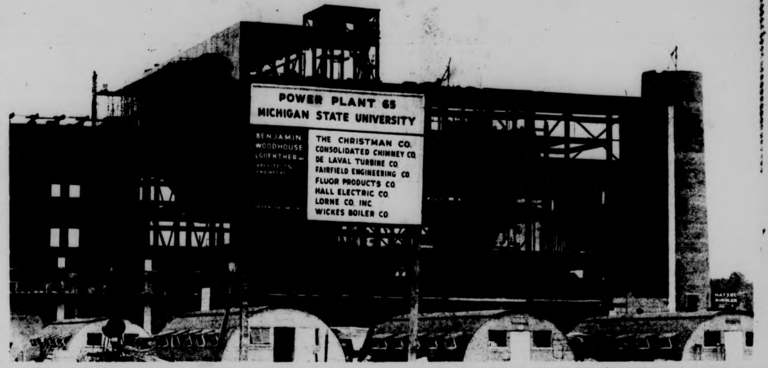
MORE POWER TO YOU: It's full steam ahead at the Stadium Road site of the new Power Plant as a fall completion is expected. Second phase of the operation
