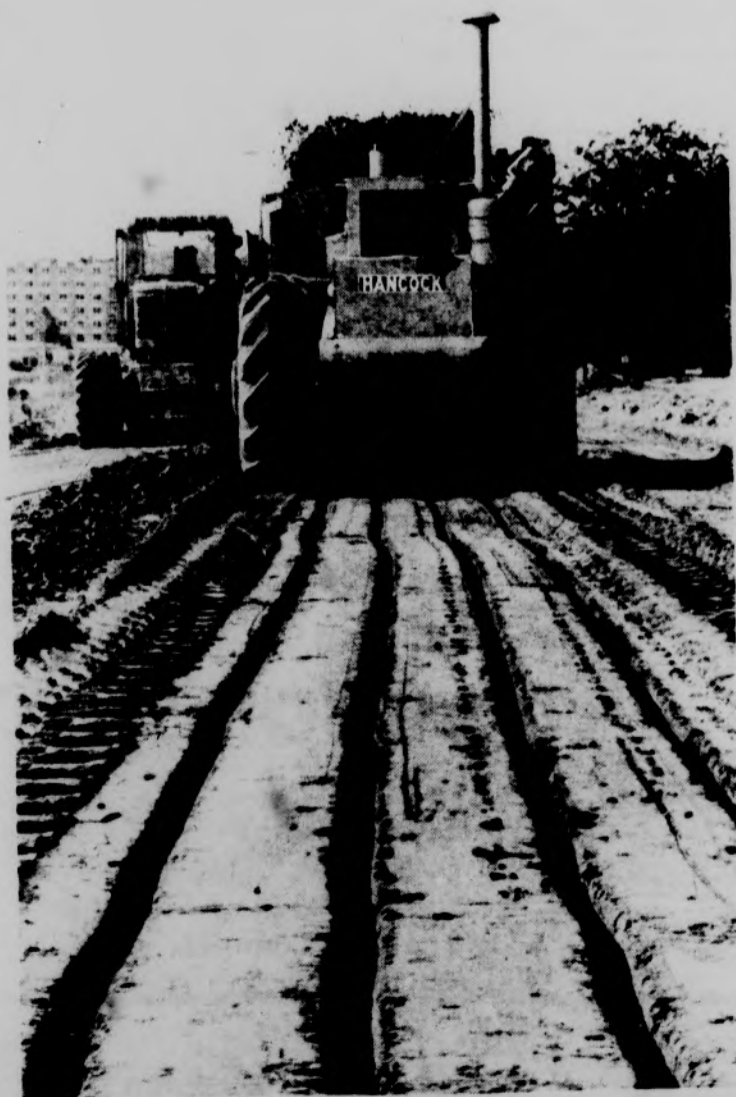
HAGADORN ROAD WIDENING--Work is now in progress to widen Hagadorn Road on the east side of campus from its present two lanes to a four lane boulevard. Photo by Cal Crane
