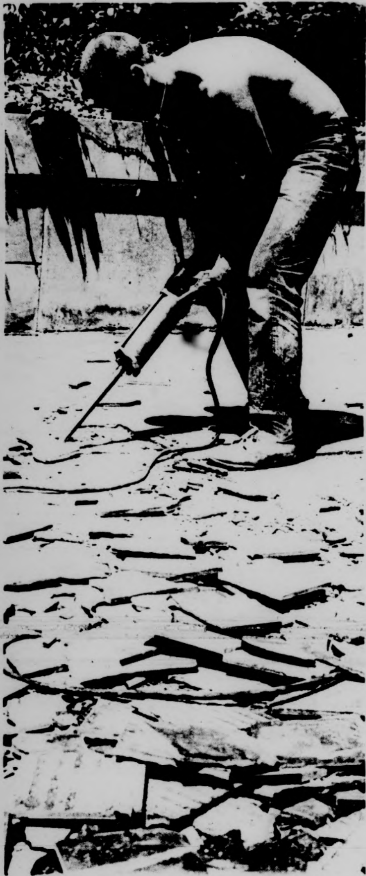
NEW UNION STEPS--Workmen took advantage of lower pedestrian traffic during the term break to replace worn tiles at the Union's West Circle Drive entrance. Maintenance work was also done on the Auditorium's steps. Photo by George Junne
