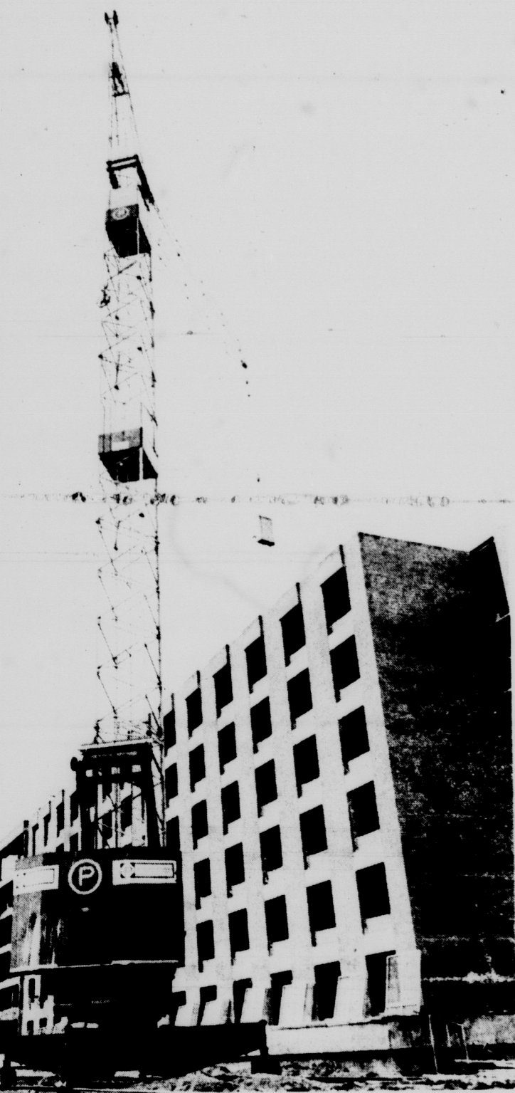
LARGEST CRANE—This crane, owned by the Granger Construction Company, is the largest of its kind in operation in the world. Photo Dave Sykes
