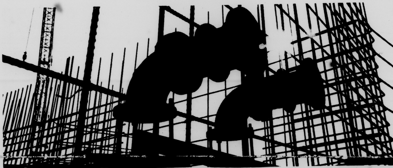
BRODY RELIEF—This is a view of the rapidly progressing sewage disposal plant being built West of Trowbridge Road and the I-496 interchange that
