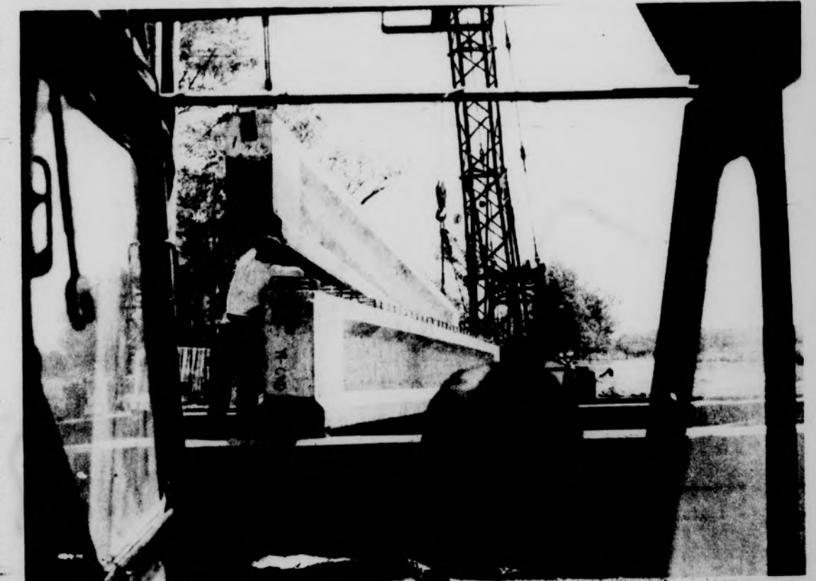
BOGUE BRIDGE PROGRESSES--Amid heated campus discussion of next year's driving regulations, the once-controversial Bogue Street Bridge continues to move toward completion. The new bridge will be a vital link in the new access route system proposed for this fall.
