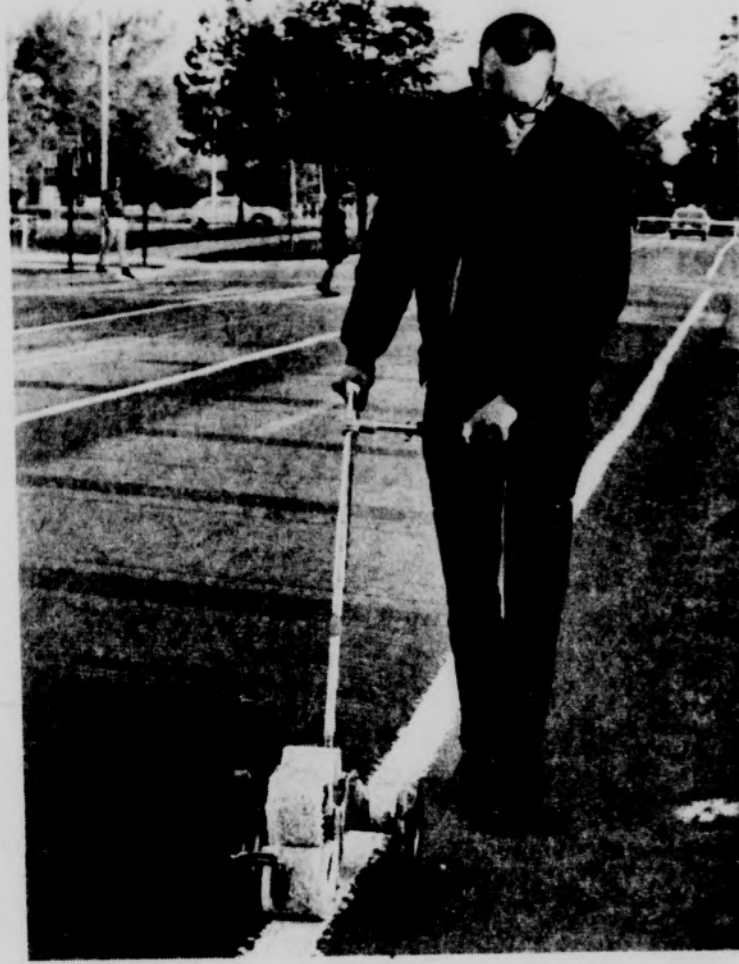
LAYING SAFETY LANES--Pete Sinclair, Hartford freshman, paints white lines on Farm Lane for the bicycle traffic lane experiment currently being conducted by University police. Photo by Jerry Carr
