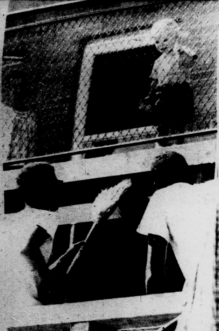
VILLAGE FIX-UP TIME --Painting, cleaning and general maintenance work is being completed by married housing maintenance crews readying the villages for fall term occupancy. Keith Williams, left, and Al Bivens, get ready to paint part of the steelwork under the watchful eye of Duane Patram, balcony supervisor. --State News Photo.
